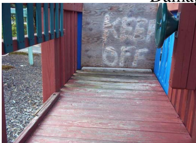
Worn Out Flooring
