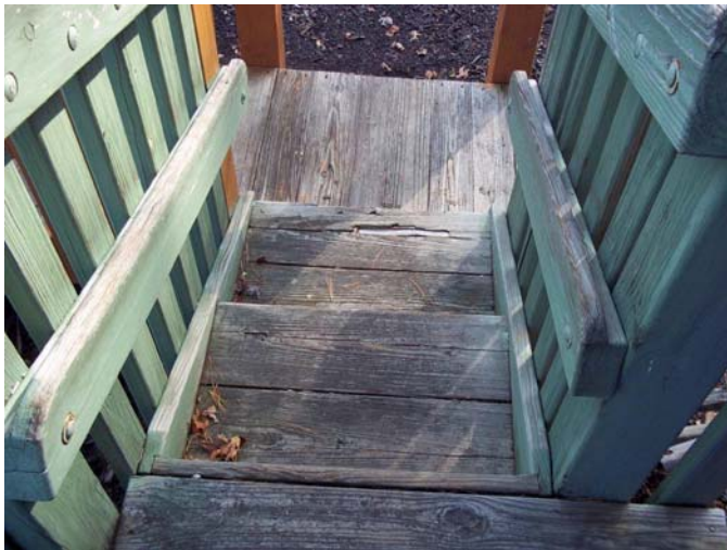
Worn Out Floor Boards
